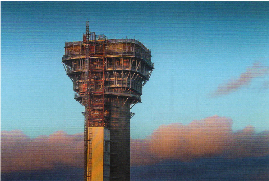
LEFT: Work to remove the 'filter gallery' at the top of the Windscale Pile reactor chimney. BELOW: A giant door frame being lifted into place at the Pile Fuel Cladding Silo - part of the process of opening up the silo to retrieve historic nuclear waste inside
